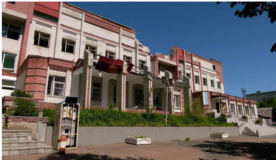
Outpatient building of the Chernihiv Central District Hospital after strikes by the Russian army in 2022. Source: Suspilne Chernihiv 76
