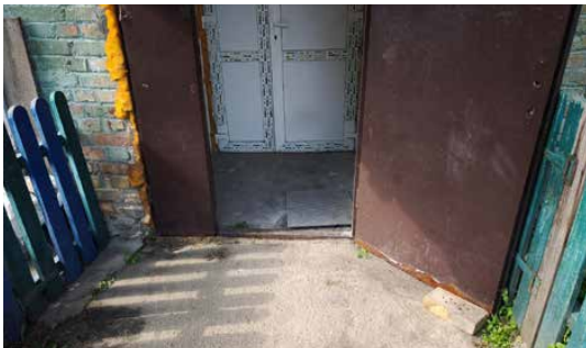
A person in a wheelchair cannot fit through such narrow doors or over the threshold. Residential building at 20a Sadova Street, Horenka, Kyiv region
