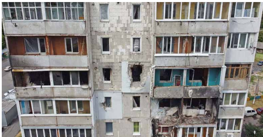
Residential building at 2 Semashka Street, Borodianka, Kyiv region. After the occupation
