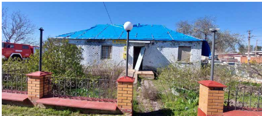
Damaged post office in the village of Posad-Pokrovske. Photo as of May 2025.
