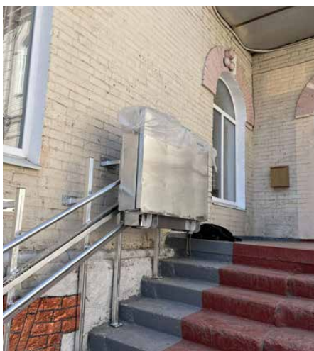
Wheelchair stairlift in the shelter at Vocational School No. 26 in Kremenchuk
